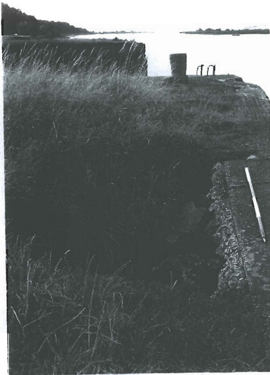
Fig. 14: Scour erosion to the harbour wall at Newburgh Photograph - Rudiger Bahr
